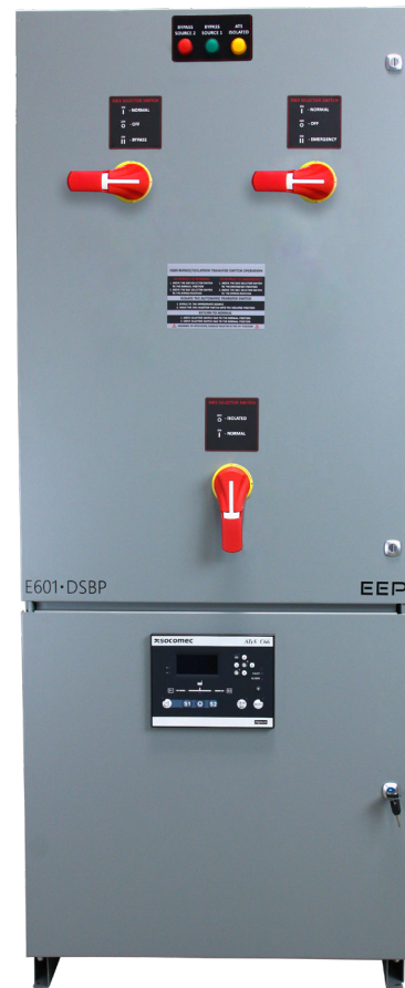
Bypass in Emergency
